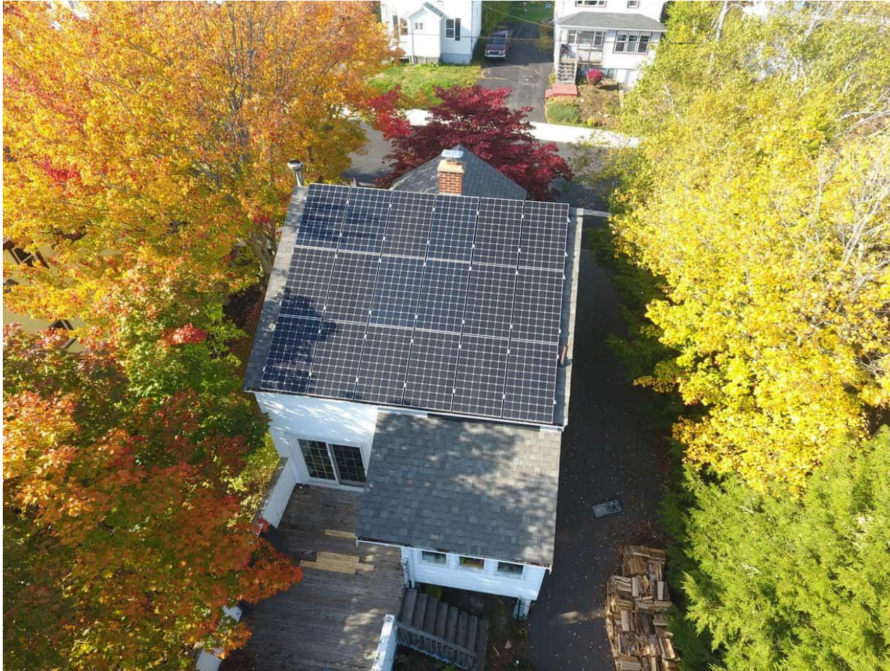
Above: A 6 kW solar home – Image: WattsUp Solar
